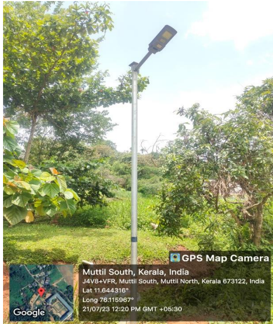
Fig-9: Solar Lamps
