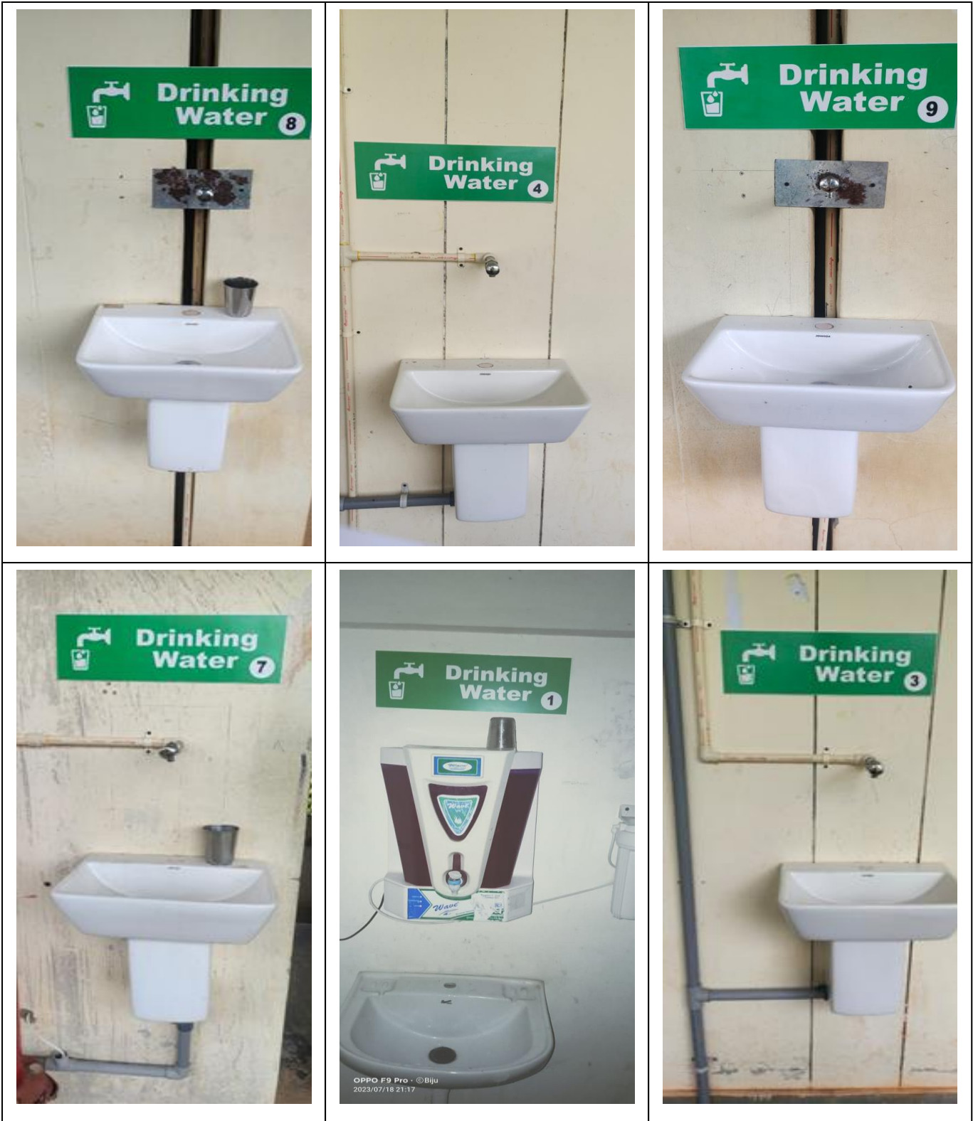
Fig-4: Drinking Water Facility
